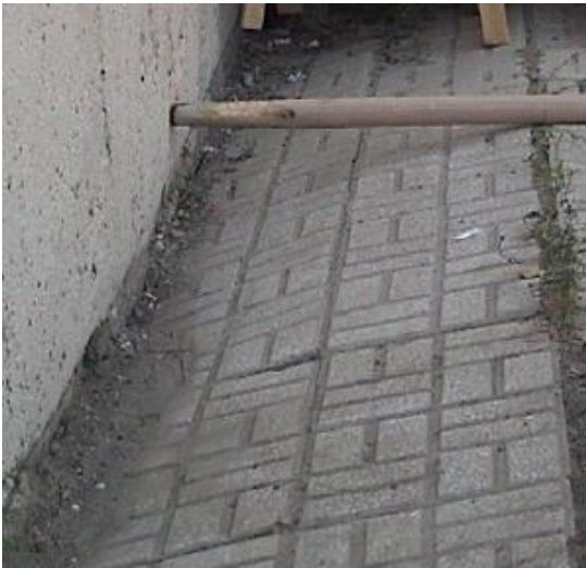
Figure 13 Damage in floor due to swelling of gypsum soil.
