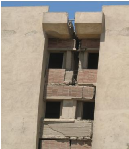
Figure 12. Rupture of beam and column near expansion joint of a reinforced concrete building in Egypt.
